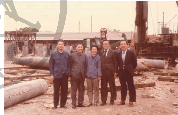
During the construction process of Jinling Hotel in the early 1980s, the Tao brothers are at the building site.
